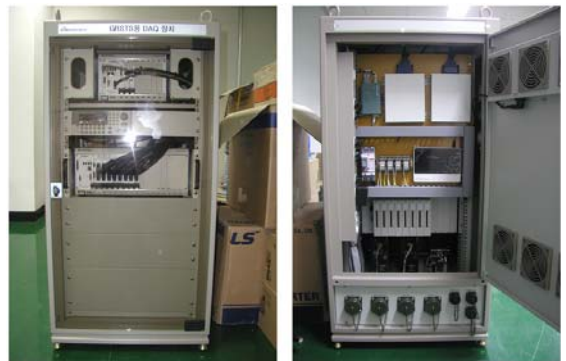
Figure 6 Control/DAQ System Rack
