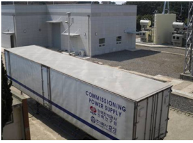
Commissioning Power Supply
