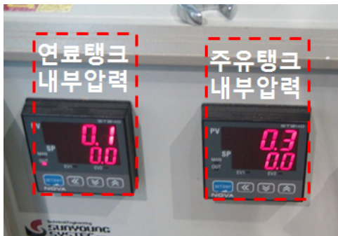
Fig. 6 Tank Pressure before Refueling
