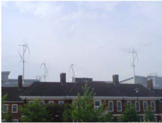
Defra, Weybourne Four turbines installed on a roof top at Defra
