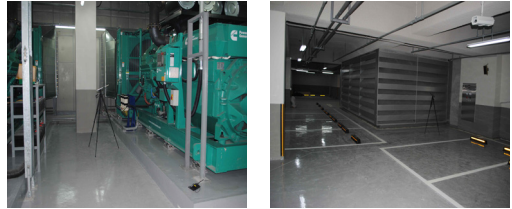
Fig. 3 Supply-return measurement photograph
