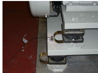
Fig.1 typical shipboard machinery with a common bed on resilient mounts
