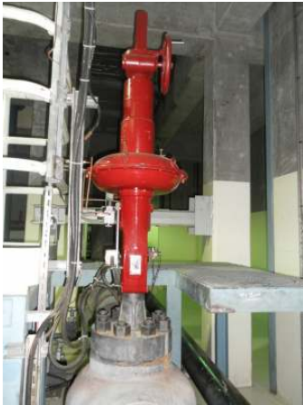
Fig 2. View of feed-water recirculation piping isolation valve
