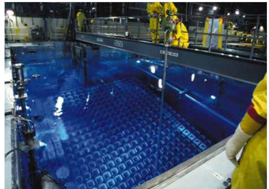
Fig.4 PWR Spent Fuel Storage Pool
