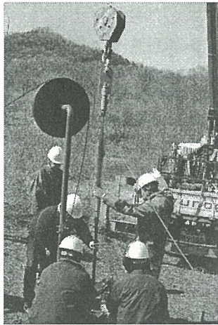
Fig. 2. Field demonstration of straddle packer system
