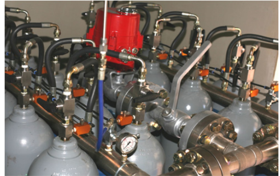
Fig. 2 High Pressure Air Storage Tank
