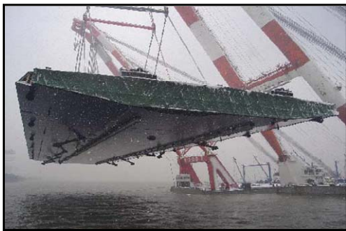
Fig. 2 Loading the heavy block of Incheon Bridge by two floating cranes (김화수 2008)
