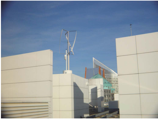
Fig. 1 Vertical wind turbine installed on top of a building.
