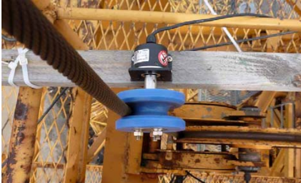
Figure 3. Encoder sensors test
