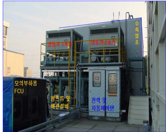
Fig. 4 Site view of cooling system.
