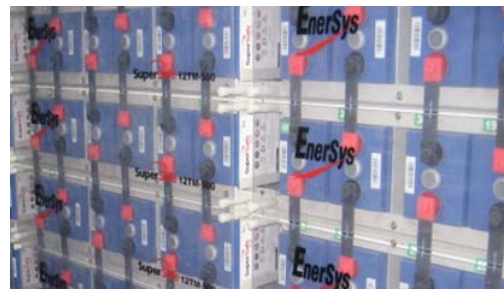
Fig. 6 Uninterrupted Power Supply.
