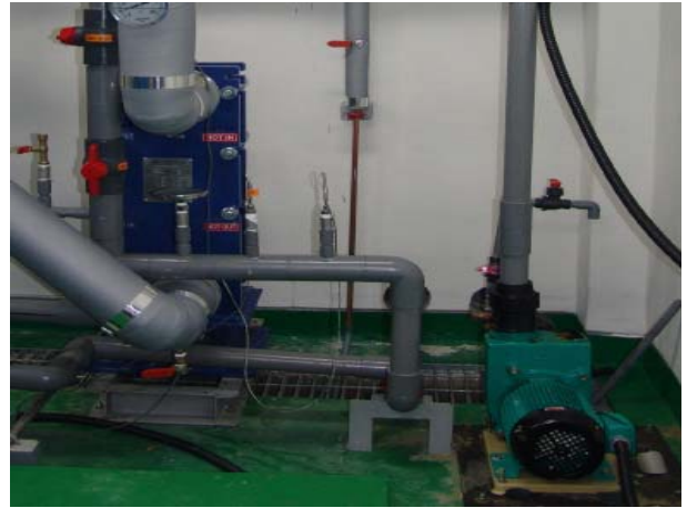
Fig. 7 Photograph of Sea water heat exchanger & pump
