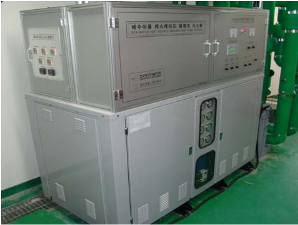
Fig. 6 Photograph of installed heat pump
