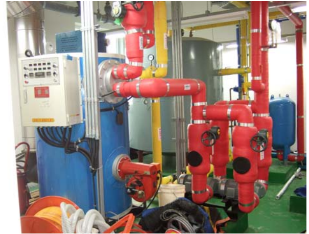
Fig. 2 Photograph of Heating equipment
