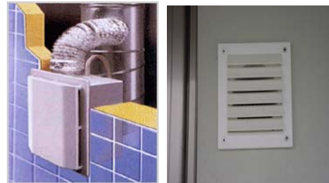
Fig. 2 Wall exhaust malodor old system
