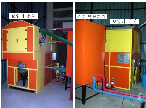
Fig. 3 Pictures of 350 kW wood pellet boiler.
