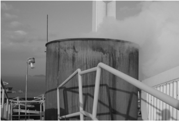
(a) View of boiler steam exhaust pipe operated
