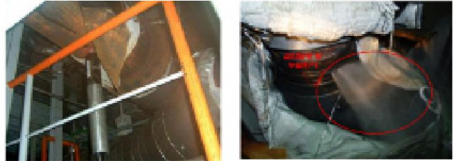
Fig. 2 Pipe crash in nuclear power plant
