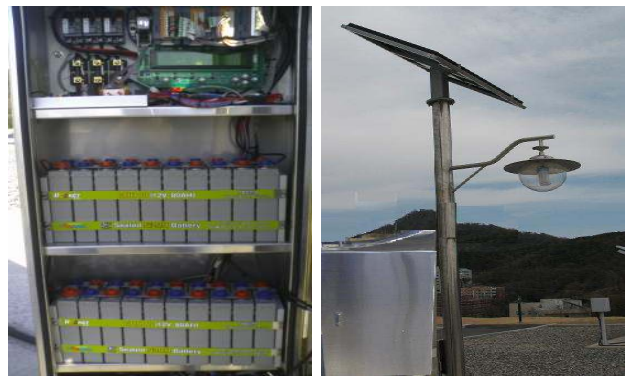
Fig. 3 Terminal box and PV system
