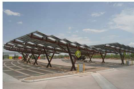
Figure 11: Springs Preserve Bifacial Fixed Installation
