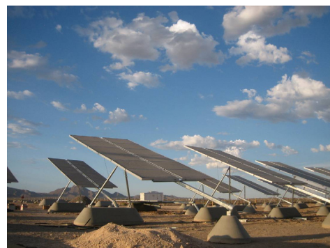
Figure 12: Nellis AFB 2.5MW Bifacial Tracker Installation
