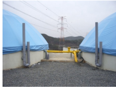
Fig. 5 Gas holder installed on the top of anaerobic digester
