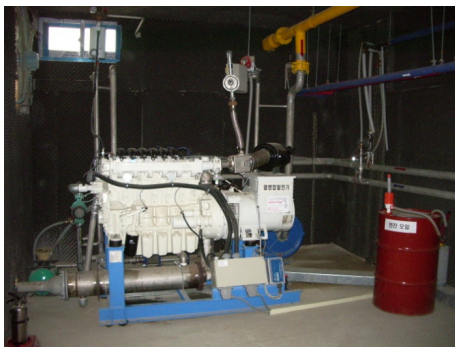
Fig. 6 The 60kW power CHP generator
