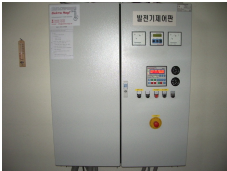
Fig. 7 Control panel of the generator
