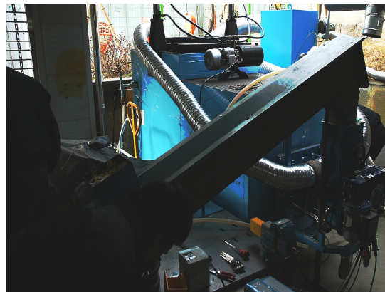
Fig. 1 Picture of the woodchip boiler
