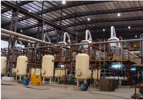
Fig. 5 Installed waste tire pyrolysis system for 120t/d treatment
