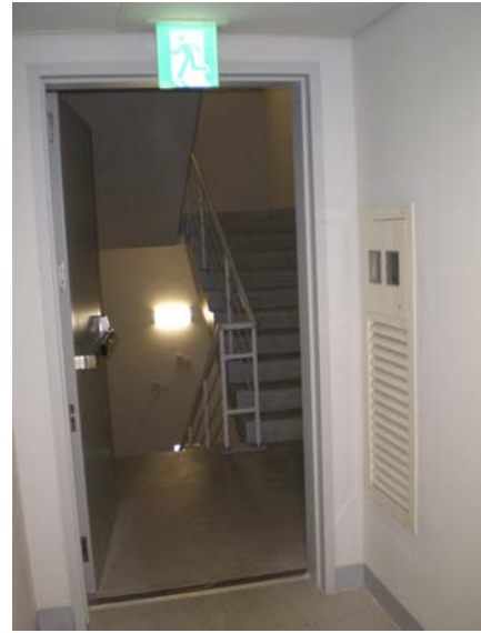
Fig. 4 Photograph of lobby and damper
