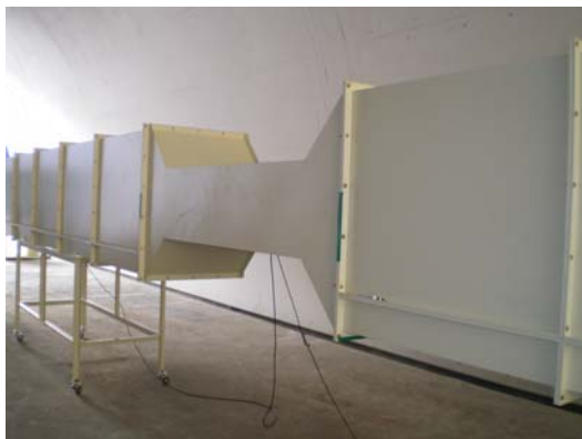
Fig. 7 Photograph of venturi-typed duct
