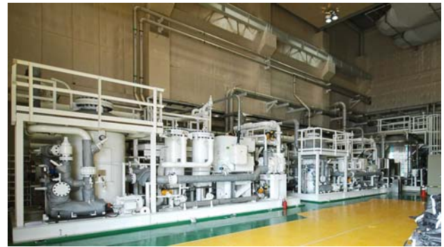
Fig. 2 Photo of the WCS installation
