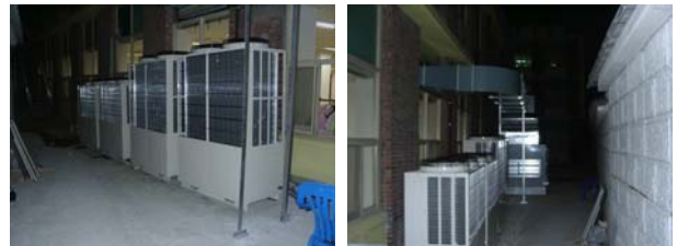
(c) Heating and cooling equipment.
