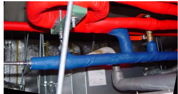
Fig. 2 Picture of facilities inside ceiling for underground shopping center.
