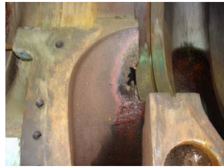
Fig. 6 Casing damaged by cavitation
