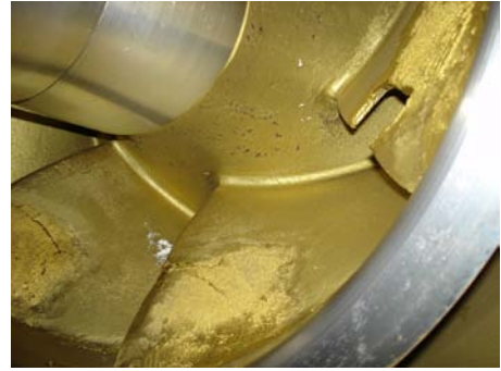
Fig. 7 Impeller damaged by cavitation
