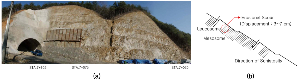
Figure 1. Cut-slope adjacent to the 00 tunnel(a) and diagram of collapsed pattern (b)
