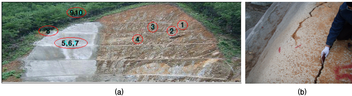
Figure 2. Cracks location on the cut-slope and tunnel portal area(a), and cracks on tunnel portal(b)
