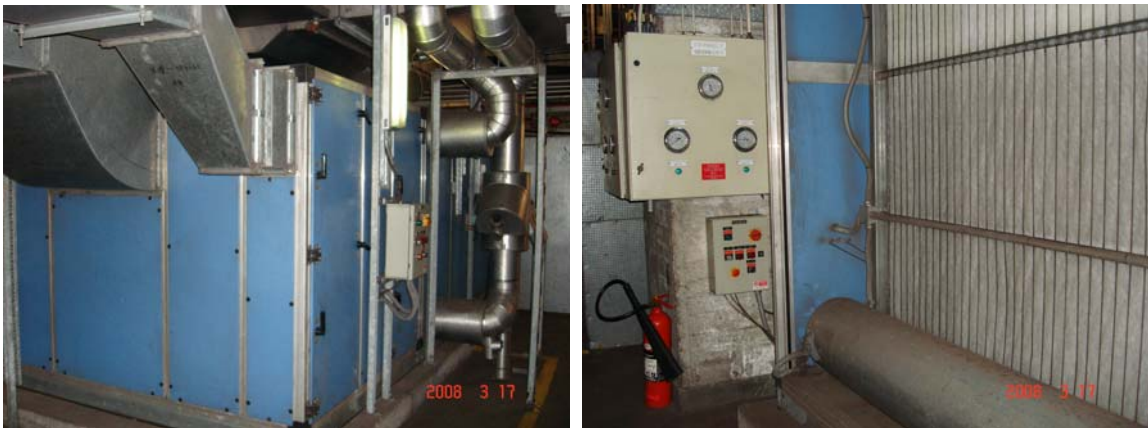
Fig. 4. Air handling unit and roll filter system at mechanical room of Choi Hung station
