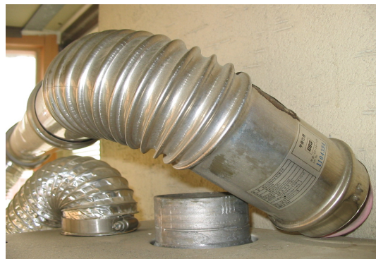
Fig. 1 Gas boiler accident by break away of exhaust pipe.
