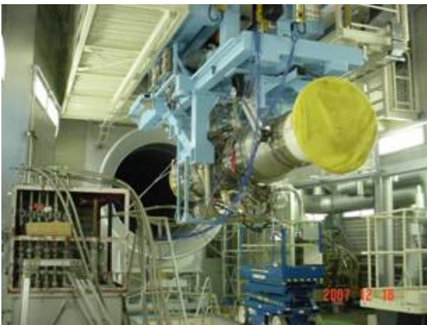
Fig. 21 ESPR engine installed into renovated engine cell
