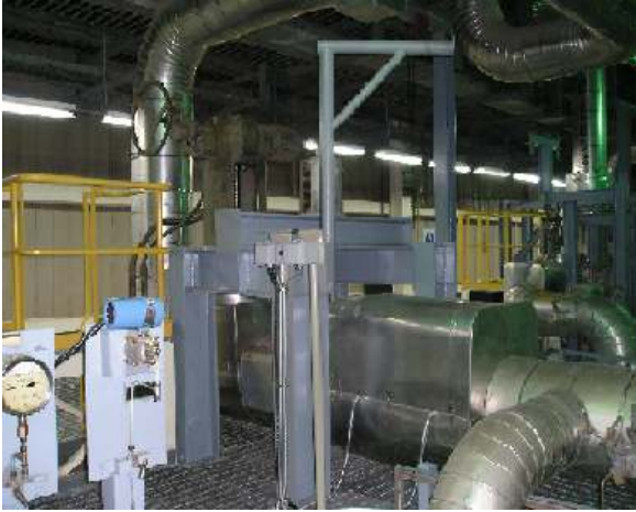
Fig. 2 Main water pump outlet check valve
