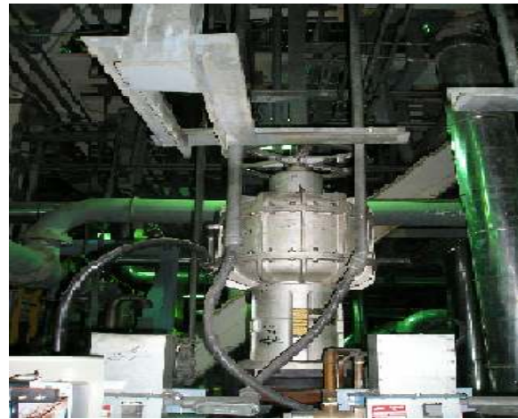
Fig. 1 Main steam dump valve
