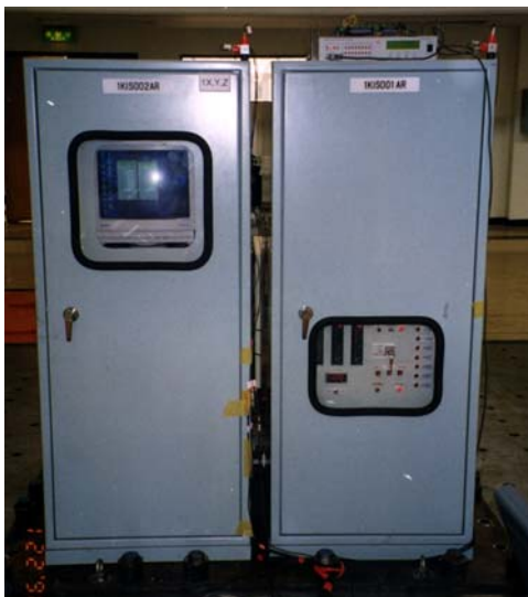
Figure 1. The test cabinet
