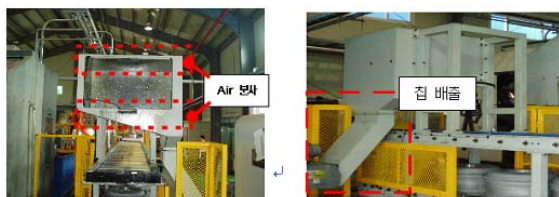
Fig. 6 Figure of Air Shower and chip remove device
