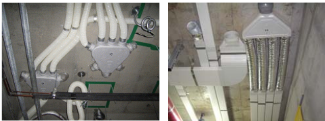
(a) Circular duct (b) Rectangular duct Fig. 1 Construction view of air distributor
