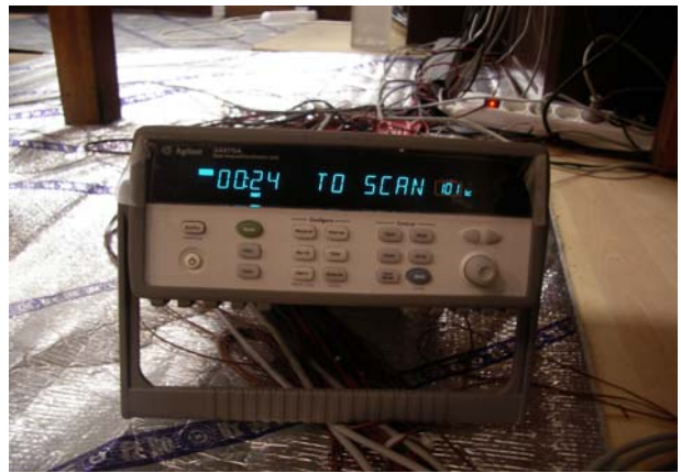
[Fig.10] View of data logging system
