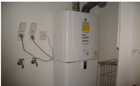
[Fig.3] Boiler for the experimental house
