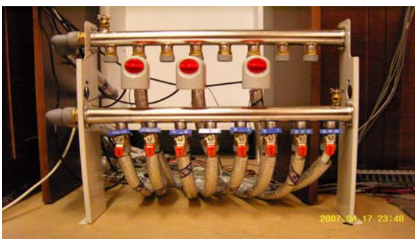
[Fig. 4] Distributor with 8 openings installed to living room
