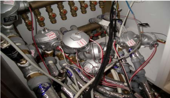
[Fig.7] Temperature and flow sensor installed to distributor
