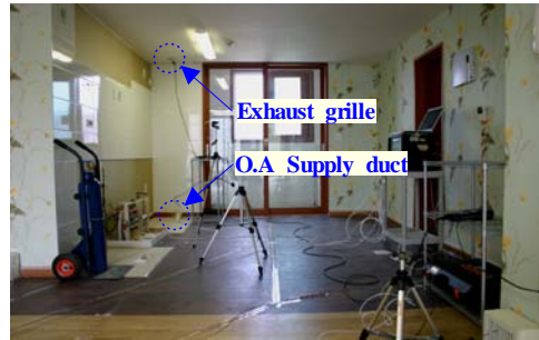
(c) Outdoor air incoming part and exhaust grille on back side
