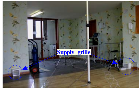
(a) Indoor air supply grille
