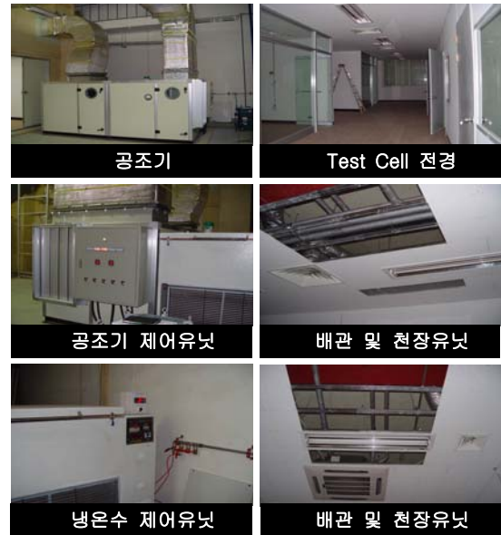
Fig. 4 HVAC simulator for experiment.
