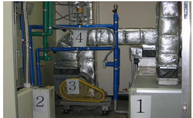
Fig. 1 Experimental apparatus of central cooling system.
