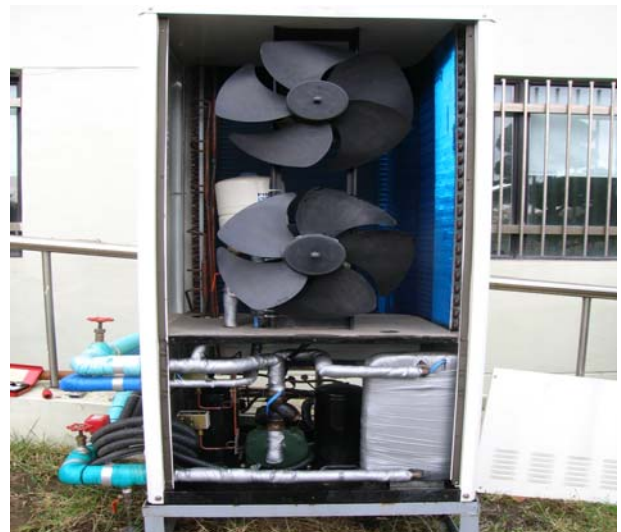
Fig. 2 Inside appearance of Chiller.
