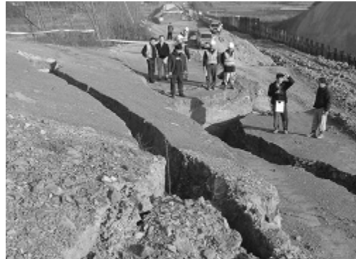
Fig. 1. Slope failure in the primary excavation stage.
