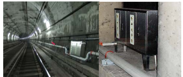
Fig. 5 Siamese connection in tunnel
