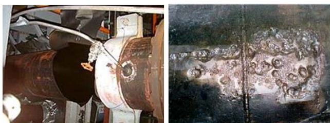
(a) The failure accident at Mihama (b) Wall-thinning pipe due to flow accelerated corrosion
