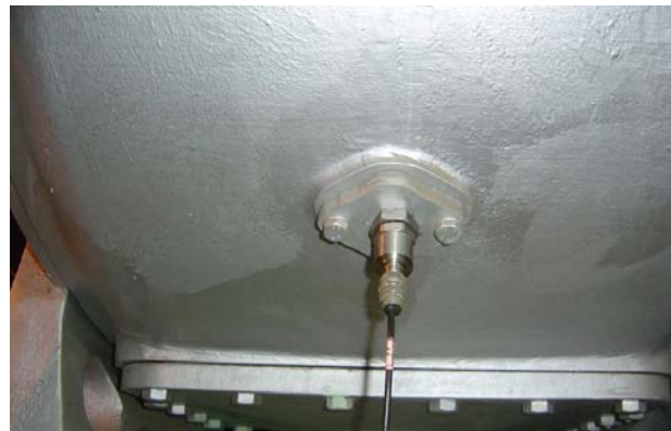
Fig. 7 Vibration measurement at core hole of turbocharger for two stroke low speed diesel engine
