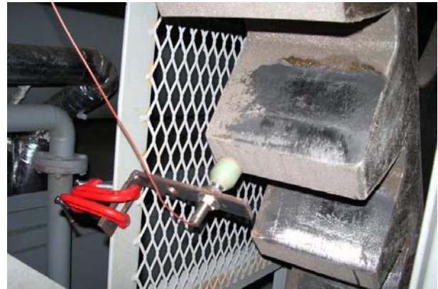
Fig. 3 Gap sensor for torsional vibration monitoring at turning wheel
