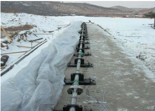
Fig. 5 Pressure pipe of the soft recovery system
