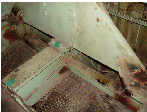
Fig 2. View of flue gas reserve support cracked
