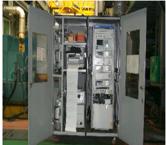
Fig. 1 Exhaust Gas Analyzer
