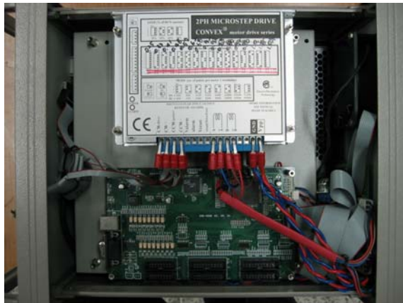
Fig. 3 The controller – Internal
